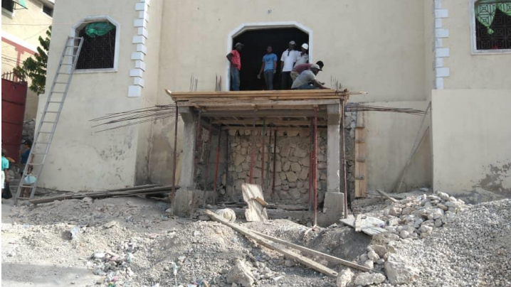
The stairs at Carrefour have to be repositioned.
