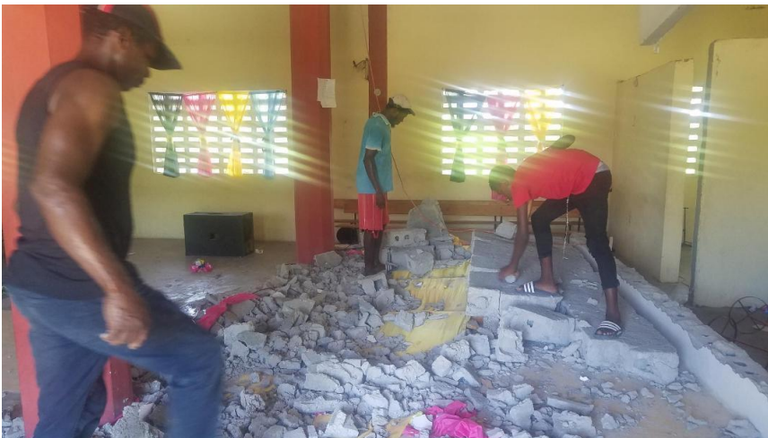
Damage at the Christville Church at Fonfrede.
